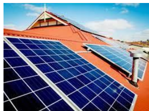
Rooftop system ~2-10 kWp
